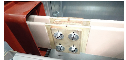
Figure 3.5. Main Bus Connection
